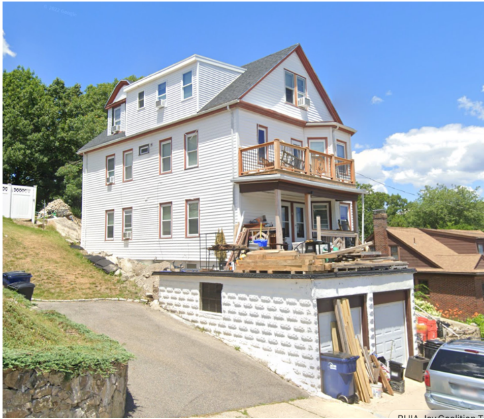
Google Street View - June 2022. Side/rear view of 7 Vershire Street showing exposed/disturbed ground and rock along portions of the building perimeter.
