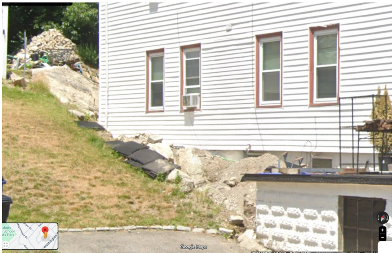
Google Street View - June 2022. Closer side view of 7 Vershire Street showing exposed/disturbed ground and rock in close proximity to the building perimeter.
